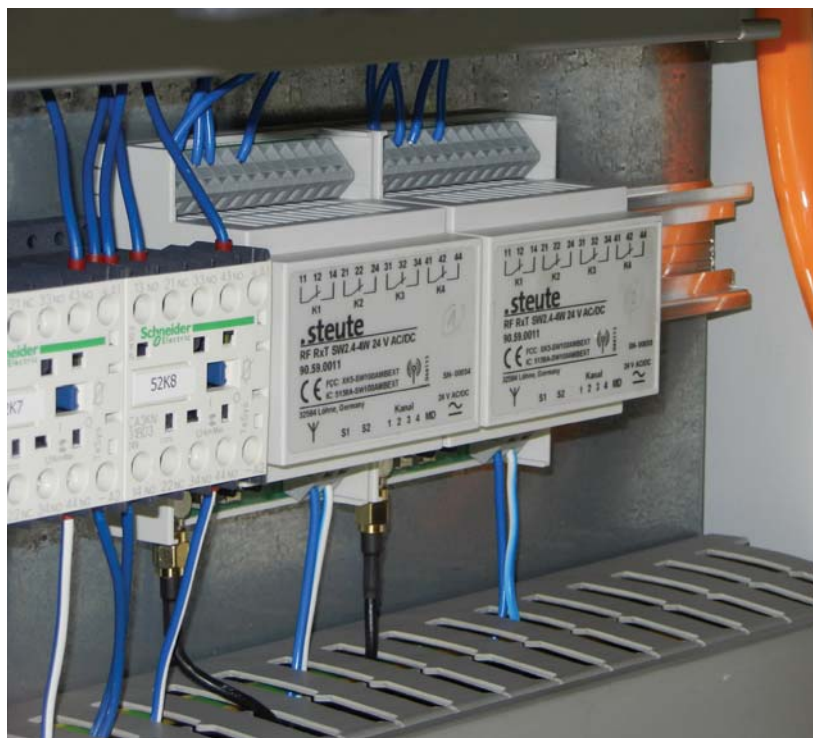
Figure 3. The receivers and evaluation units of the two wireless foot controls are installed inside the control cabinet
