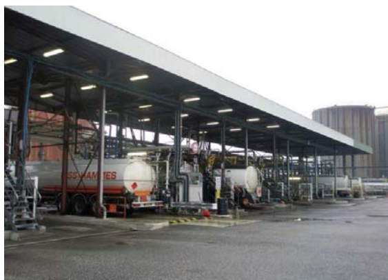
Figure 8. Application example – tank truck filler pipe position monitoring
